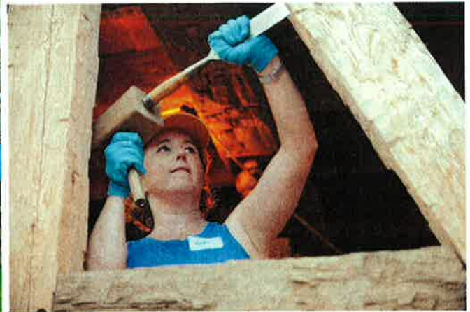
THE LUTZE HOUSEBARN (left), built in 1849, is the only remaining structure of its type in the United States. Below, Heather Lamb chisels notches for staves into a hand-hewn beam.
